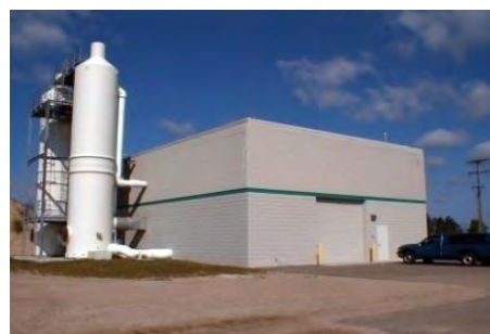
LDFA Water Treatment Facility
