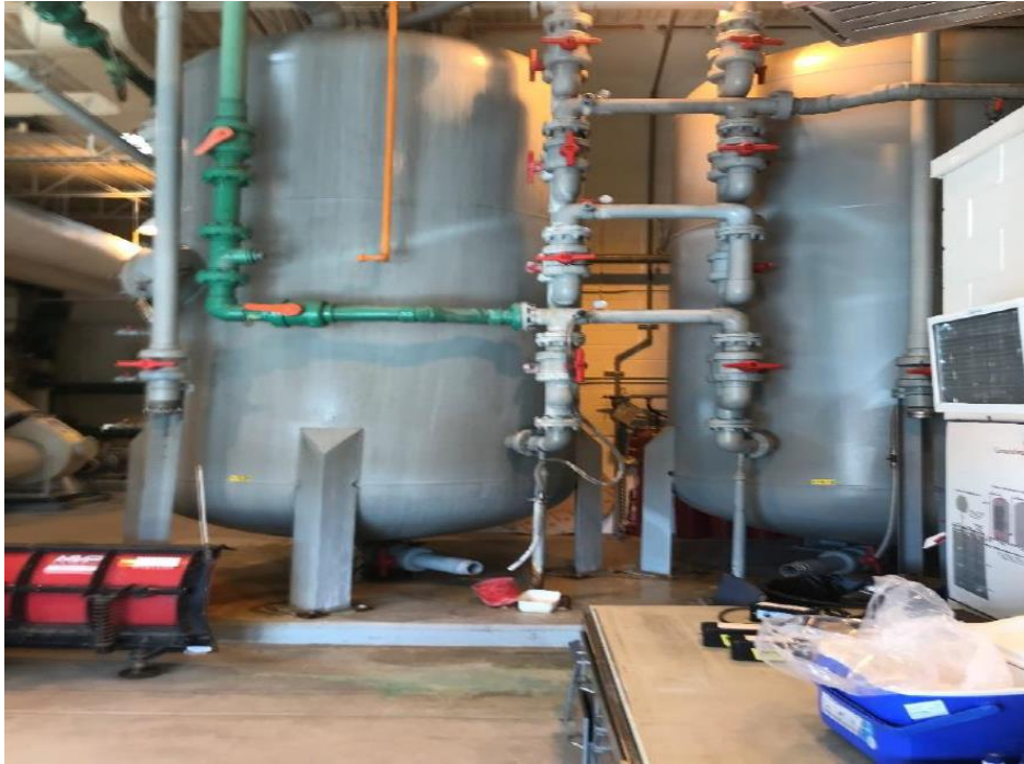
Two carbon tanks that were designed to treat hexavalent chromium from the Northernnaire Site.
