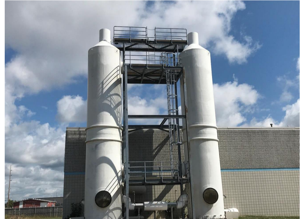
View of the two-stage air stripping system that removes VOCs from groundwater.
